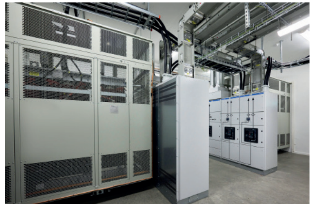
One of three transformer rooms, with two transformers and their low voltage switchgear supplying electricity for ventilation and operating the servers.
