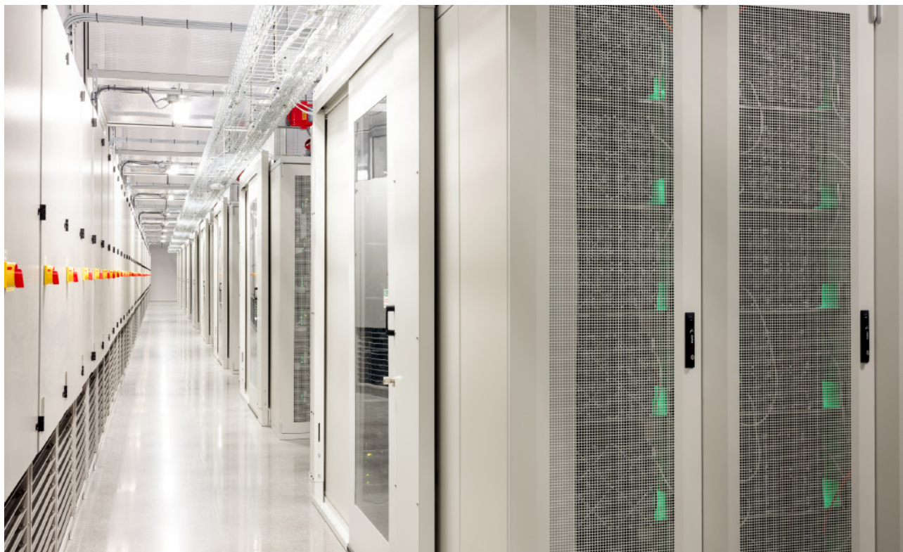
Hydro66 offers a range of services via its data center in Boden.
