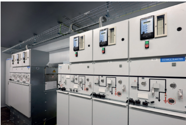
Medium voltage switchgear, 22 kV.
