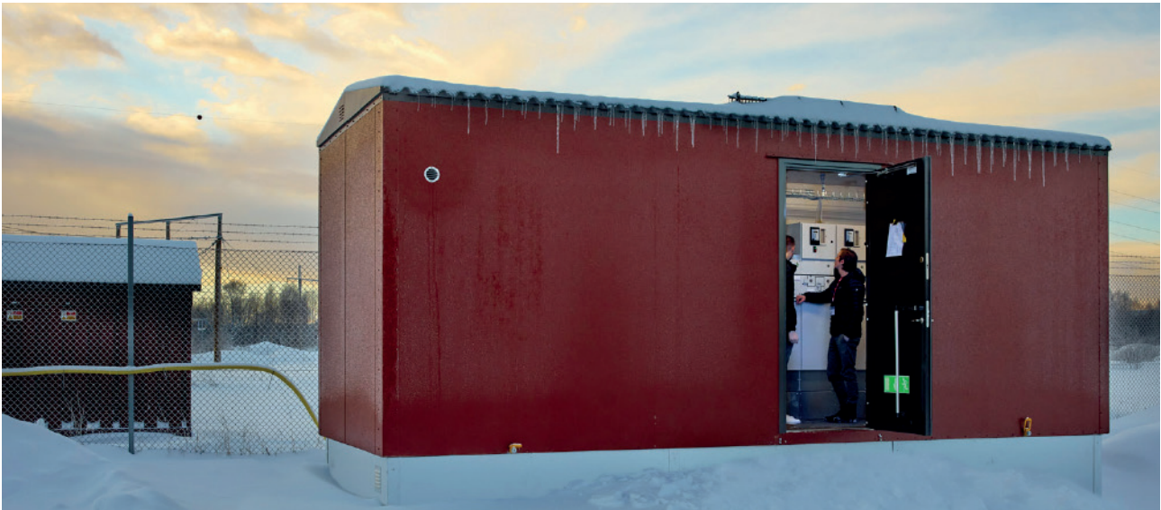
Technical shelter with medium voltage switchgear and battery equipment from Harju Elekter. Distribution from Boden Energi can be seen in the background.
