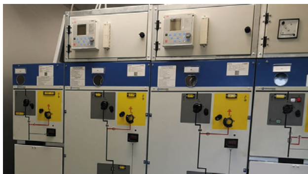
Medium voltage switchgear, CGM.3, 33 kV with ventilator.
