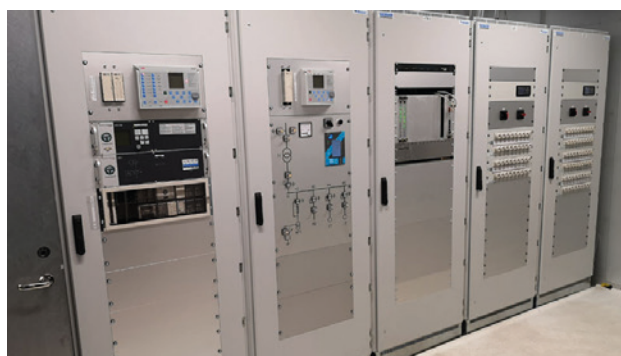
Relay SCADA system and Elcover low voltage switchgear.
