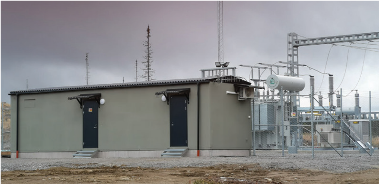
Transformer station for Härjeån Energi and Bröcklingberget wind park, north of Orsa.
