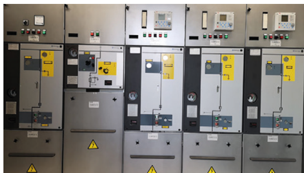
Medium voltage switchgear, CPG, 33 kV.
