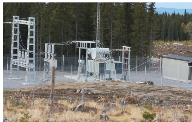
Station for connection of wind power, 45-33 kV.
