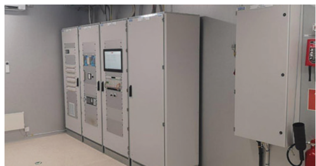
Control cabinet and local distribution board.
