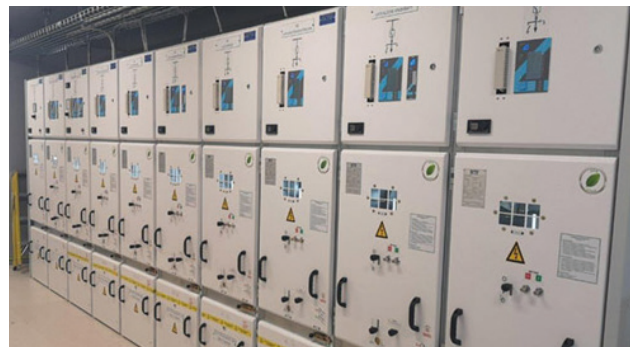
Medium voltage switchgear, SNC 10 kV.
