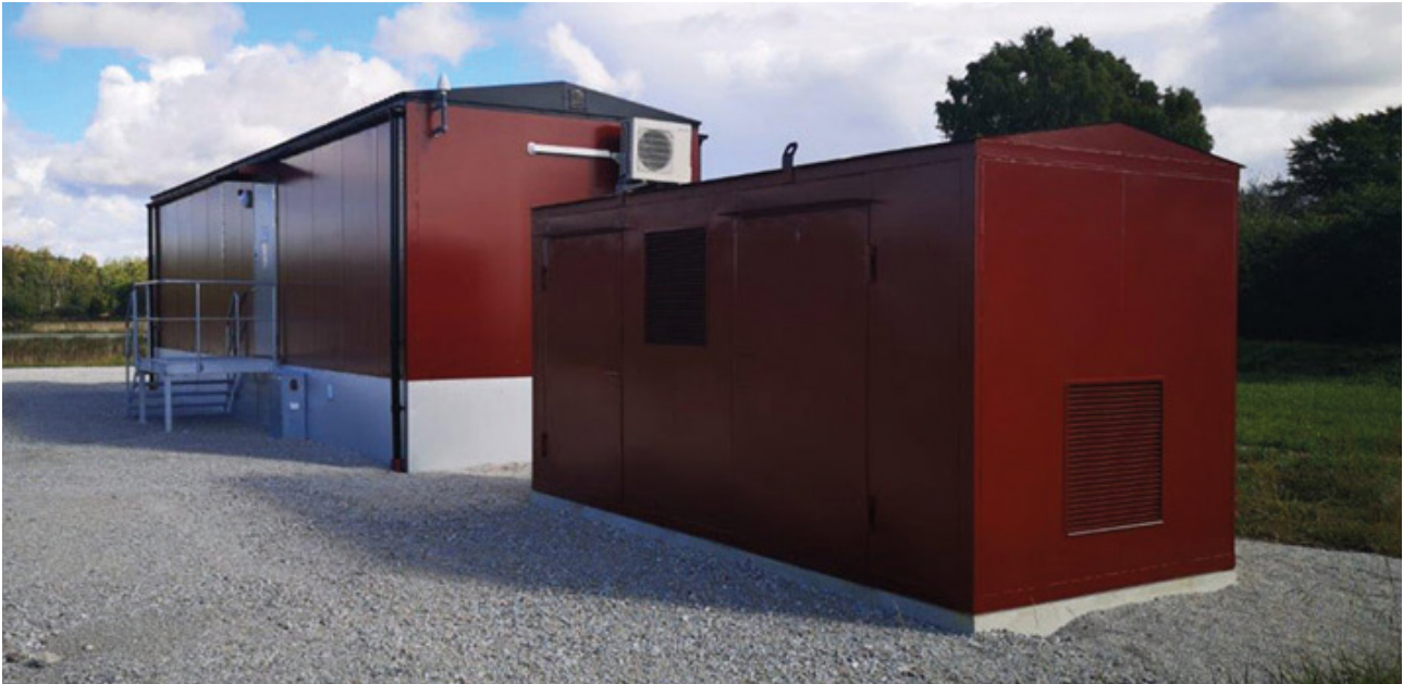
New transformer station for GEAB, Gotlands Energi, at Stenbro on the island of Gotland.
