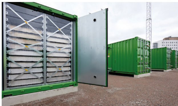
Battery storage in containers from Alfen.
