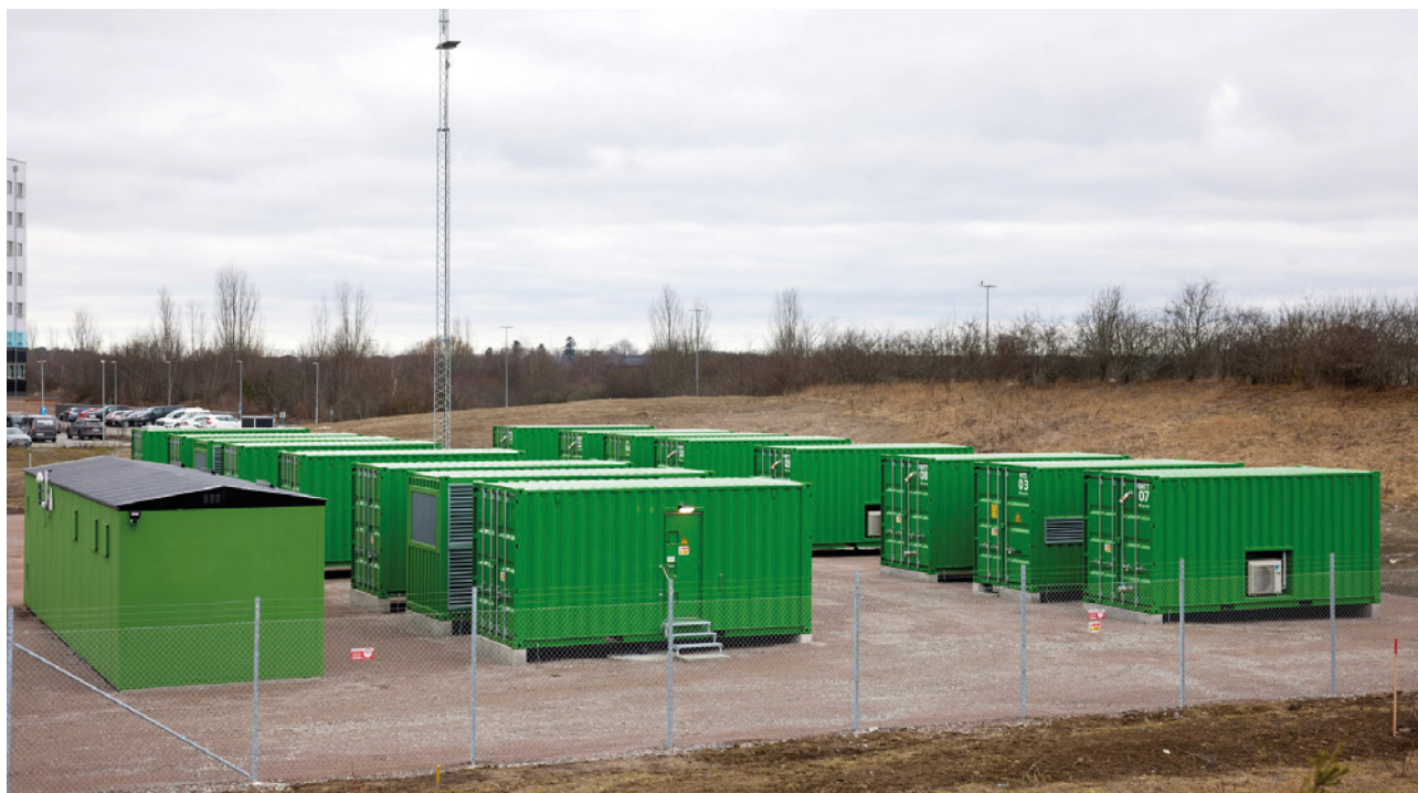
The battery storage park is equivalent in area to half a football pitch.
