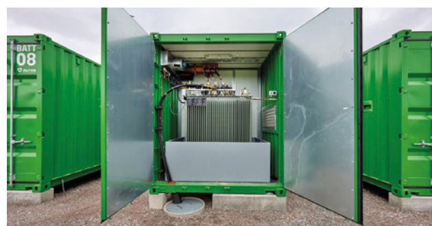
Back-up transformer, 250 kVA.
