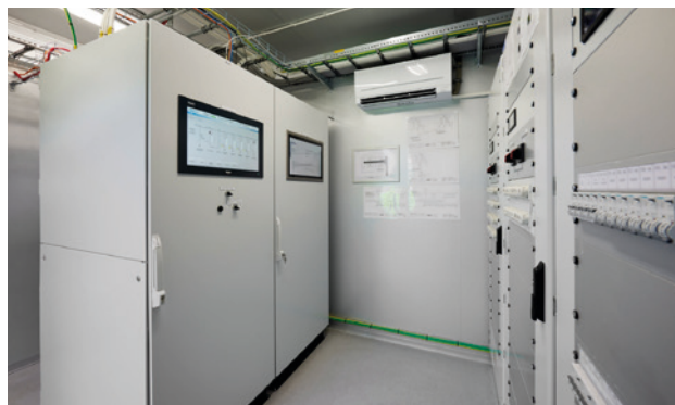
Harju Elekter's scope of supply has included switchgear and SCADA systems.
