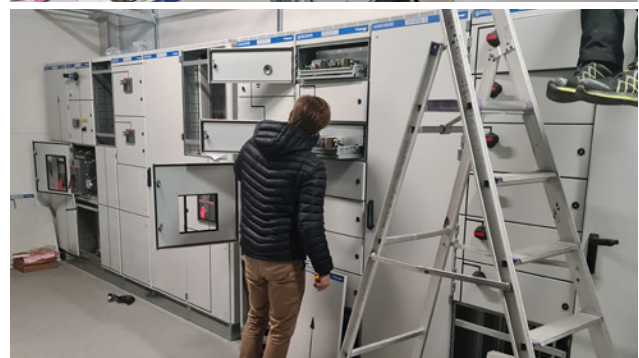
Elcover switchgear being installed at the "Thermos" in Luleå.
